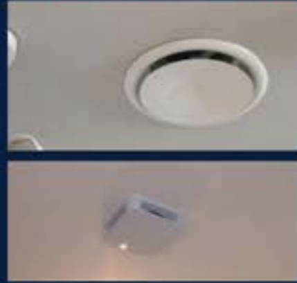
Air valves in hallway or each room?
